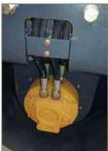
Lubrication point on each cylinder and Poclairn drive motors
